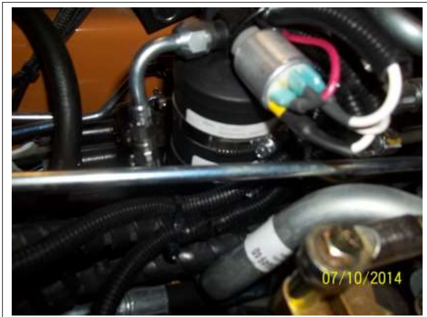
Picture of the wires at the trinary switch. FYI The trinary switch allows the condenser fans to run only when pressure builds higher to minimize power requirements.
