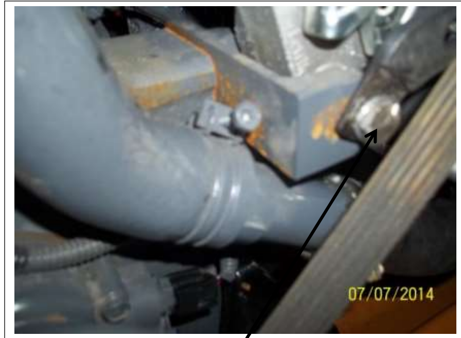
New bolt and compressor tightener bracket installed. This bolt has been cut down.
