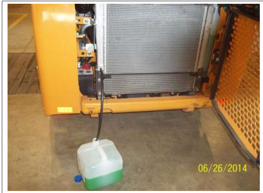
Drain radiator and engine of coolant
