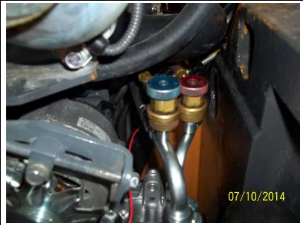
Hose connected at the compressor Picture show gauges connected to the access ports
