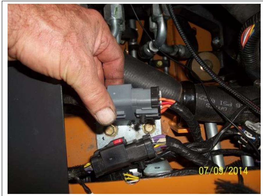
A closer look at the grey disconnect which we require to connect to separated from the other disconnects in the same area.
